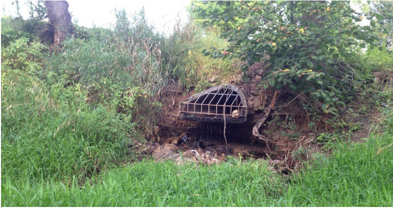
Figure 3. Erosion at existing flared end section near the #16 Green
