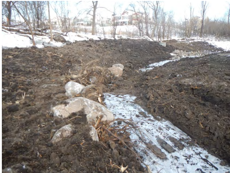
Installed root wads in the foreground. Graded banks with floodplain adjacent to the channel. New manhole and flared end section in the background.
