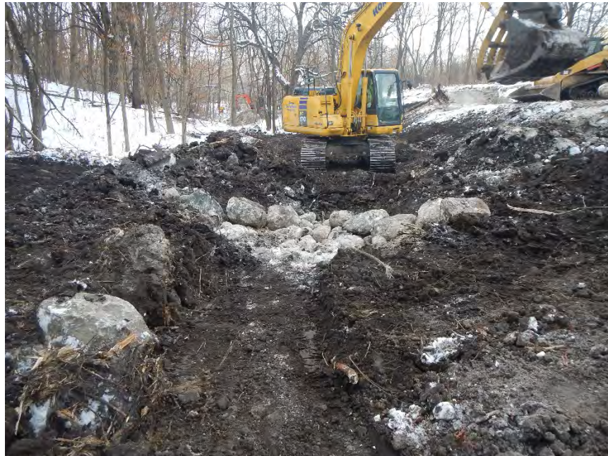
Installing a cross vane at the downstream end of a constructed riffle
