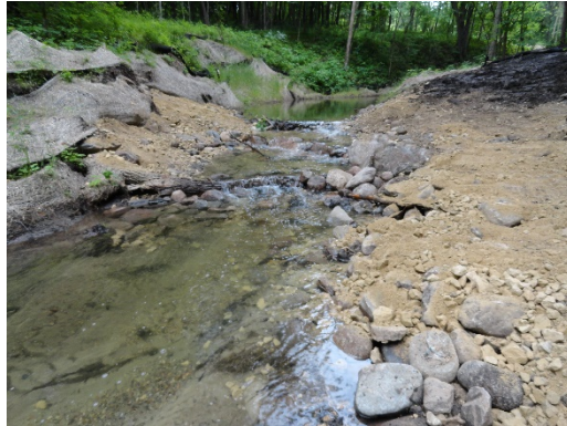
Example boulder/log cross vane modifications as a result of June 17 th site walk.
