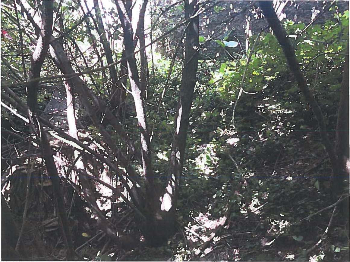
Picture 6: South side of box culvert, east bank of Riley Creek (Existing slope – 2.6H:1V)
