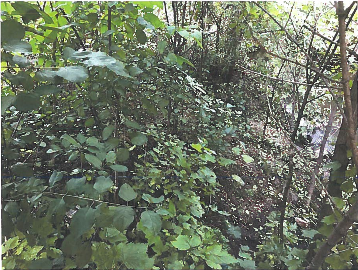
Picture 4: North side of box culvert, west bank of Riley Creek (Existing slope – 2.7H:1V)
